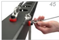
Fig. 45. - 46. Installing the left outrigger-rope (the one with the turnbuckle) for lateral bracing
